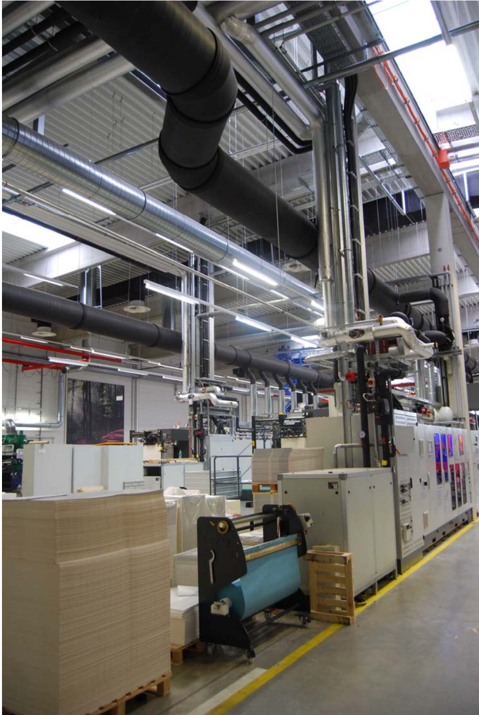
Image 2: The heated cooling water and the usable exhaust air are directed past a heat exchanger to a central buffer storage tank.
